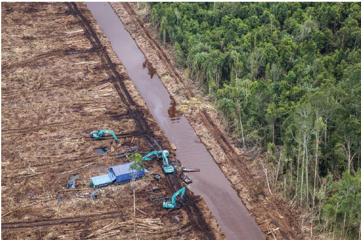
Figure 43. In May 2014, excavators worked near a recently deforested area in the concession area of PT Riau Andalan Pulp & Paper, APRIL's largest wood supplier, in Riau Province.
