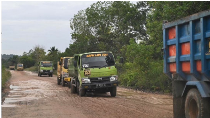
Figure 30. Trucks transporting landfill to the construction site of PT Phoenix International Resources in December 2022.
